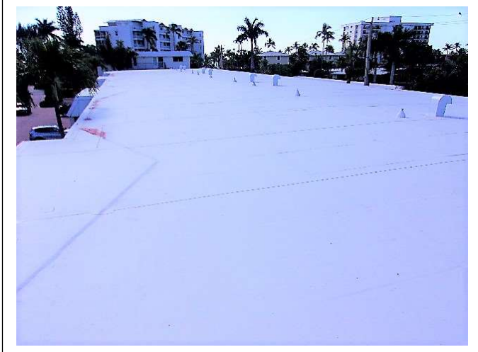
ROOF COVERING SYSTEM – The roof covering system is fully functional with no observable deficiencies.
