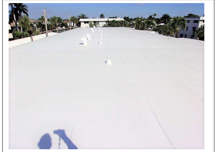
ROOF COVERING SYSTEM – The roof covering system is fully functional with no observable deficiencies.
